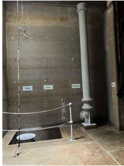
Figure 3. Internal Pipework Painting and Signage including Column Markers
