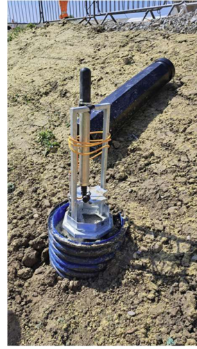
Figure 5b Data Logger stored in a telemetry pillar
