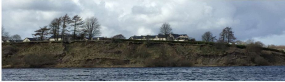
Figure 2. Erosion identified at Burgage More prior to remediation works
