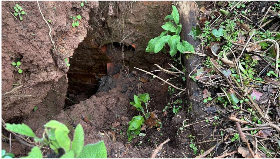
Figure 6. Clay pipe opening below the spillway, within the void. The void extended over 2.5m upstream, to the left of the image. The broken, active PVC pipe was obscured and buried within the sunken fill and not observed until it started running during the repair works.
