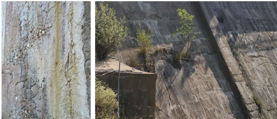
Figure 4. Damage to the dam face caused by freeze–thaw action and tree growth
