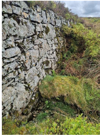
Figure 6. Dam wall viewed from downstream, showing area of leakage at the dam toe
