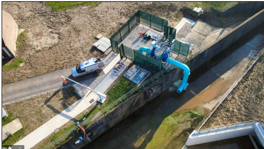
Figure 5: Uprated Outlet works (R09)
