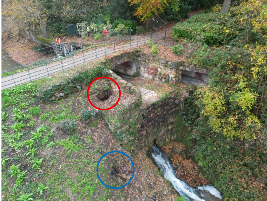
Figure 4. Daylighting void adjacent to right spillway wall, downstream of crest. Primary voiding circled red, secondary depression circled blue. Flows from the outlet chamber 'grotto' can be seen entering the streambed.
