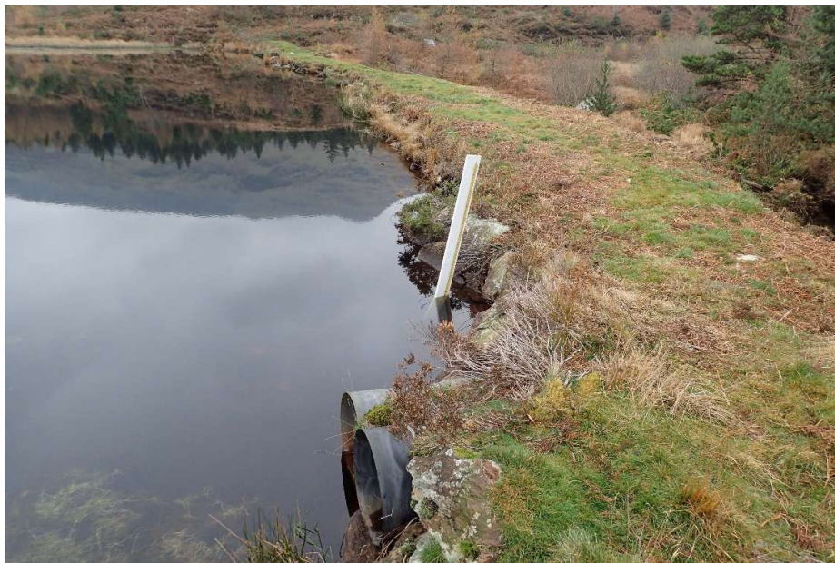
Figure 5. Example of inadequate overflow arrangement and freeboard
