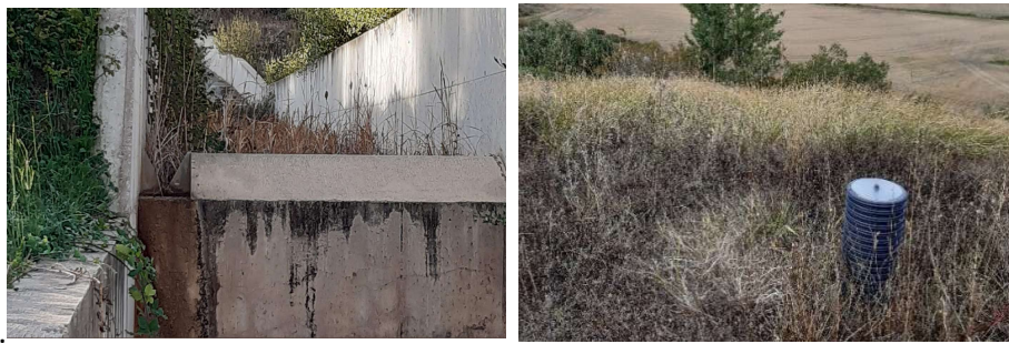
Figure 12. Examples of non-operational monitoring.
