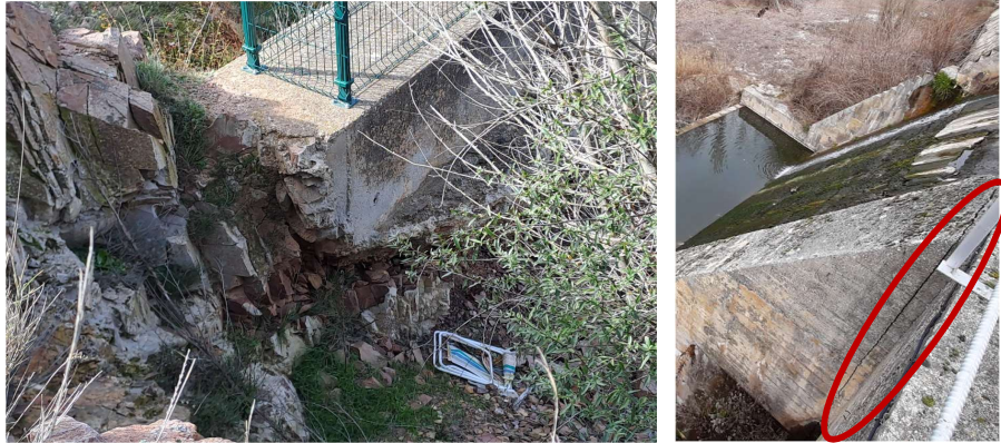
Figure 3. Inadequate abutment support and longitudinal cracking in the spillway
