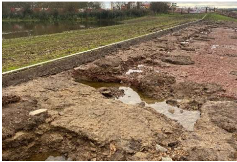
Figure 4. Isle Spillway erosion following the October 2024 events.
