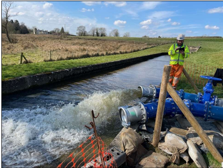
Figure 9. The outlet of the syphon during discharge
