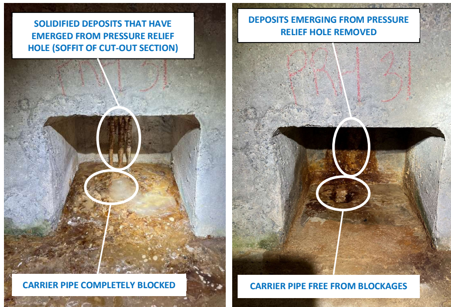
Figure 4. An example of a blocked pressure relief hole prior to cleaning works.
