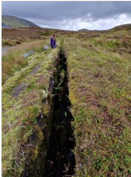
Figure 5. Dam crest viewed from the right abutment in 2025, with missing peat core
