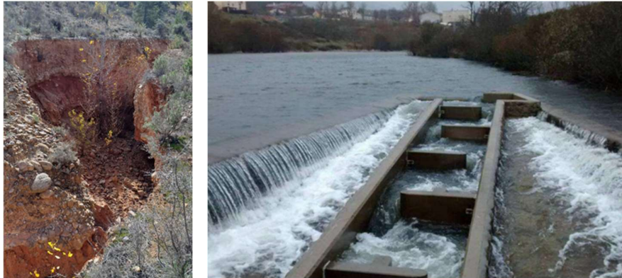
Figure 9. Erosion of the spillway and presence of a “foreign object” within the spillway
