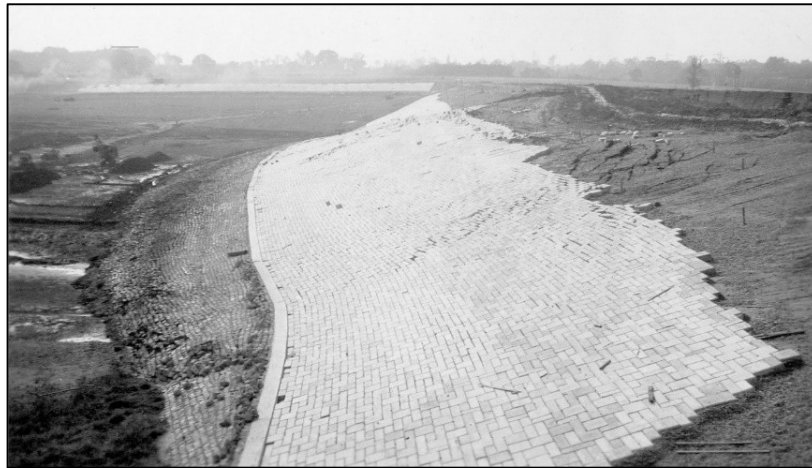
Figure 2. General view of 'original' dam failure
