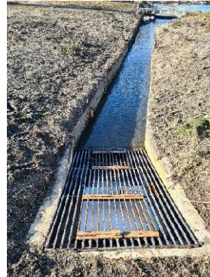
Figure 7 – Outlet screen and sloping penstock
