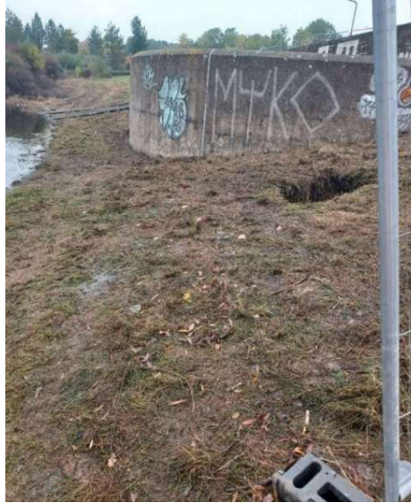
Figure 5 – Sinkhole at location of whirlpool
