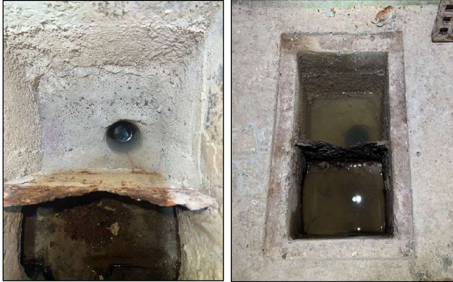
Figure 8. Relief drain No.40 prior to cleaning (left) and post cleaning (right)
