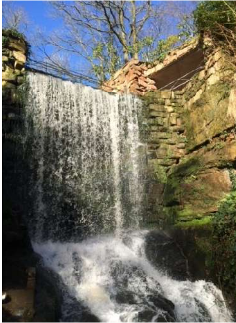
Figure 2. Overflow channel in operation as a cascade.
