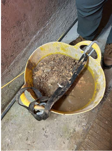
Figure 9. Example of solids removed from the drainage system
