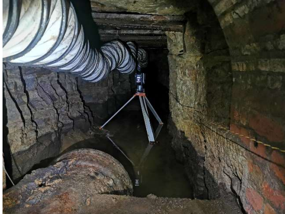
Figure 2. View of pipe inlet and weir. Note standing water on the invert of the adit.
