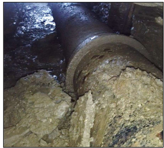
Figure 9. Minor roof fall after drilling of hole.
