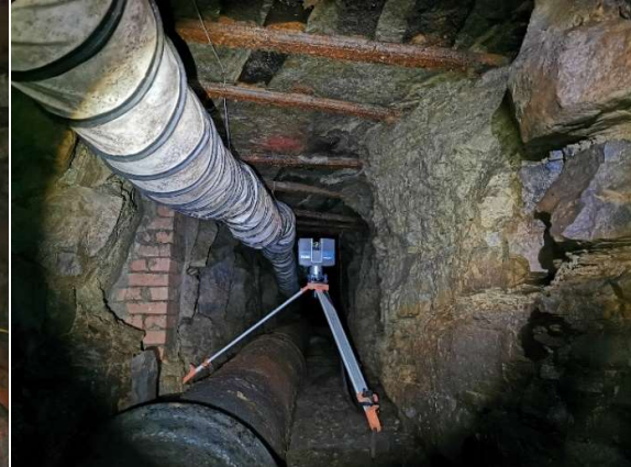
Figure 3. View in the unlined section of the adit. Notice the beams across the soffit.
