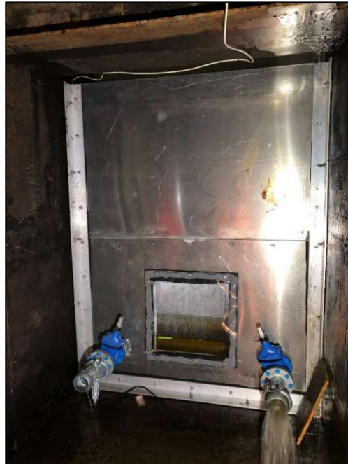
Figure 6. Scour Bulkhead – leakage monitoring station. Note window for visual check
