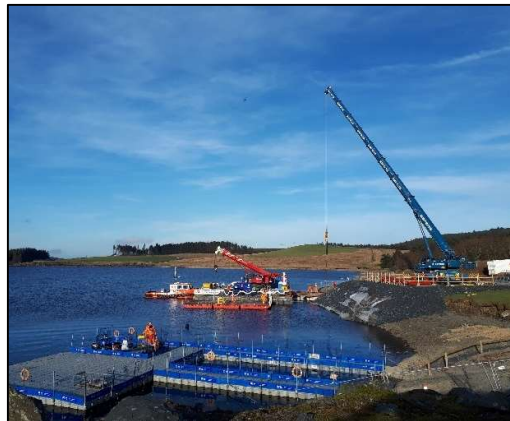
Figure 2. Temporary quay constructed to allow installation of pontoons and lifting apparatus (MMB)
