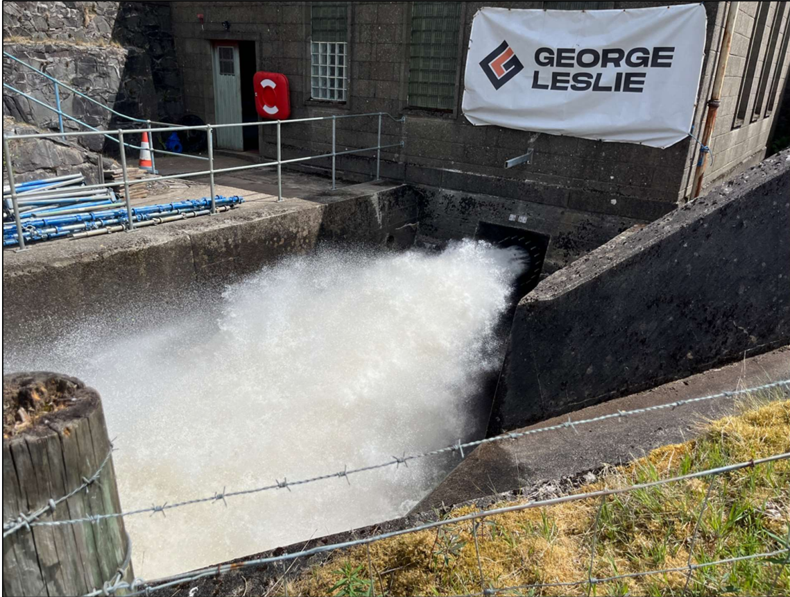
Figure 8. Needle Valve in operation in foundation of turbine building
