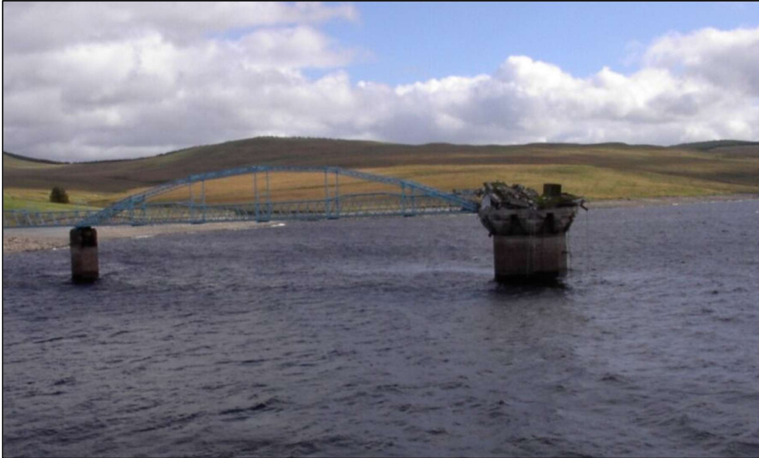
Figure 3. Valve Tower House Collapse
