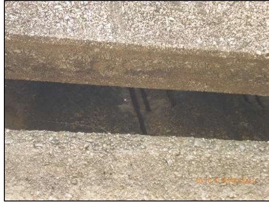
Figure 5. Rebar corrosion in air intake
