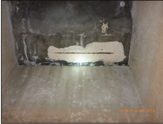
Figure 4. Spalling on siphon roof, view from siphon inlet.
