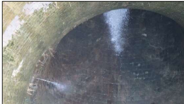
Figure 3. Leakages seen from footbridge
