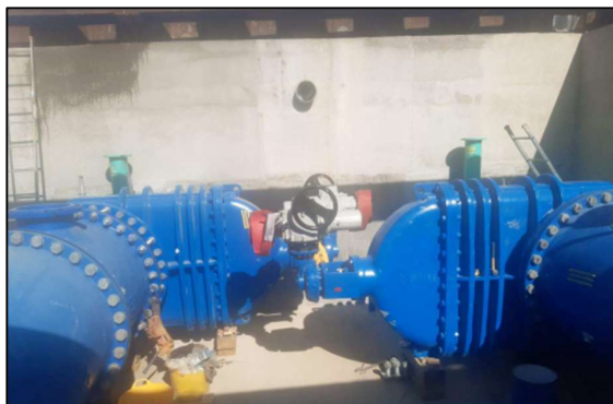
Figure 10. Crest valves showing horizontal and staggered orientation
