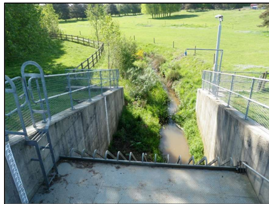
Figure 3. Sediment build up at Rase South control structure
