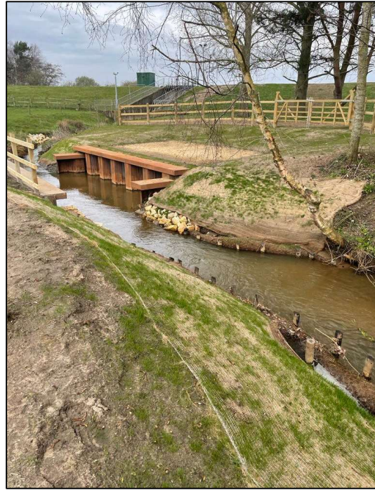
Figure 10b. Rase South in-channel chamber looking downstream (NFM upstream of the chamber)
