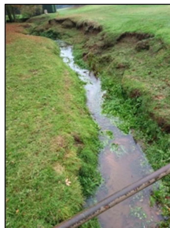
Figure 5. Undercutting of both banks along River Rase
