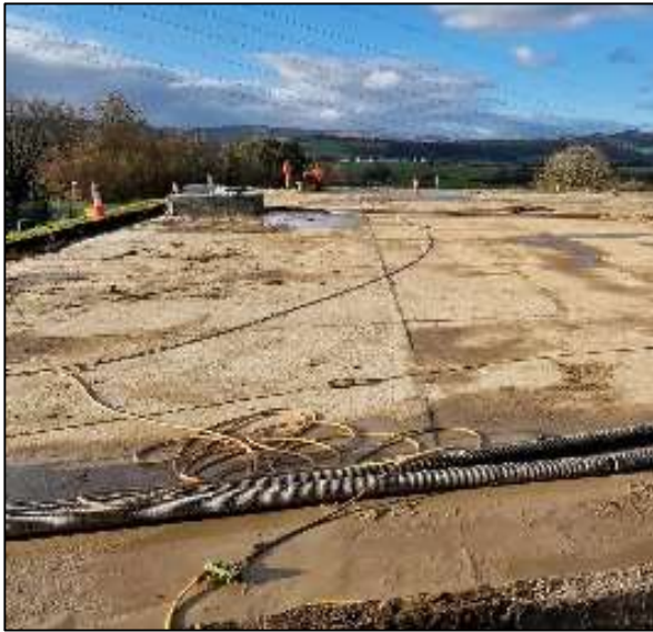
Figure 3. The exposed roof slab at Sluvad No.2. (Courtesy of DCWW).
