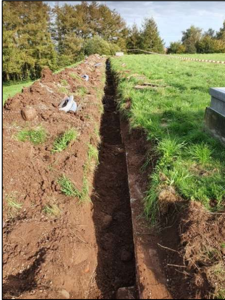
Figure 1. Excavation of the roof / wall joint at Radyr SRV. (Courtesy of DCWW).
