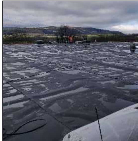
Figure 4. The new roof membrane being installed at Sluvad No.2. (Courtesy of DCWW).
