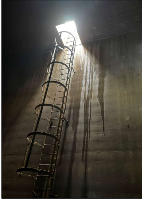
Figure 5. Roof ingress at Tongwynlais No.2. (Courtesy of DCWW).
