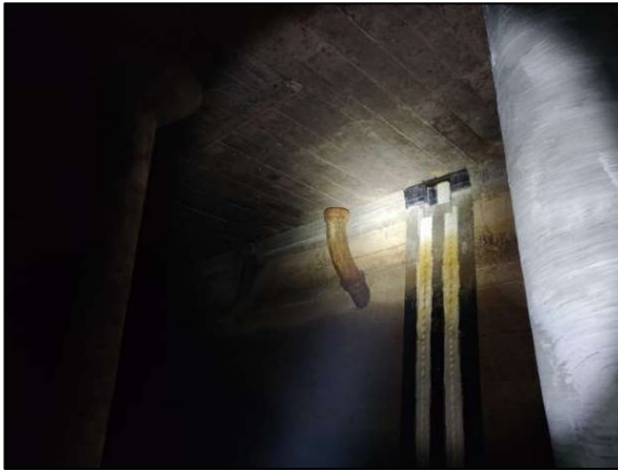
Figure 7. The overflow at Stumpy SRV. (Courtesy of DCWW).
