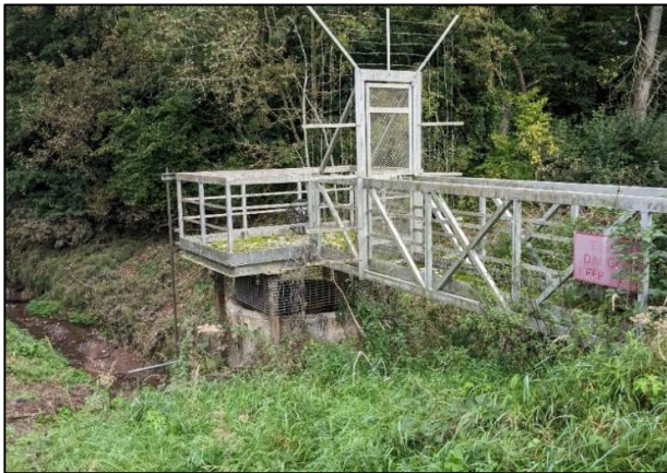
Figure 3. Photo showing overgrown condition of upstream face and overflow structure
