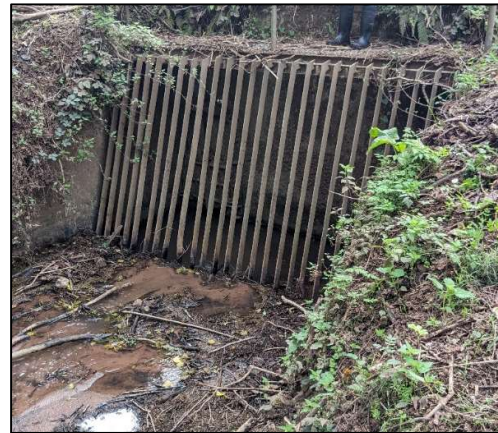
Figure 4. Photo of bar screen over inlet works prone to blockage.
