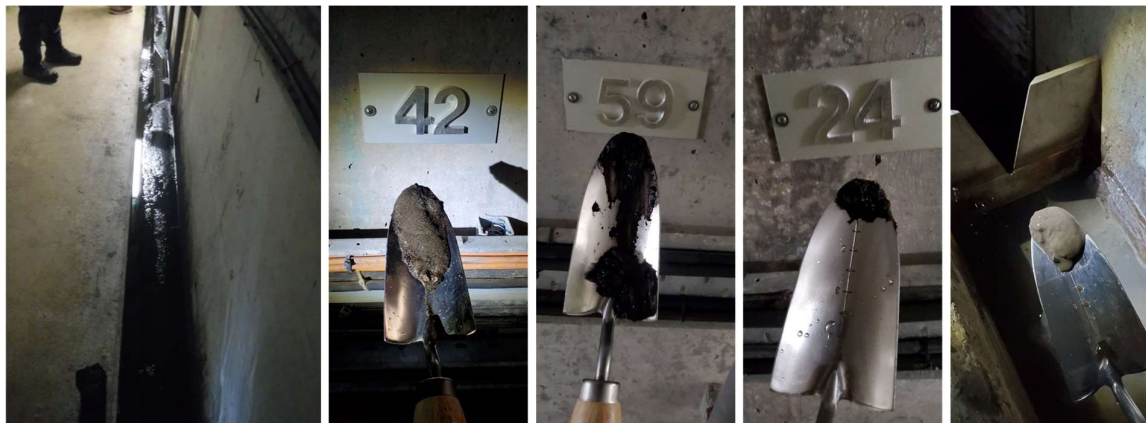
Figure 4. Photographs of dark sediments along the drainage channel
