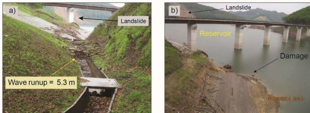
Figure 5. a): Surveyed wave runup point in the banks of the reservoir due to the landslide-generated waves. b): A photo showing damage due to the landslide-generated waves.
