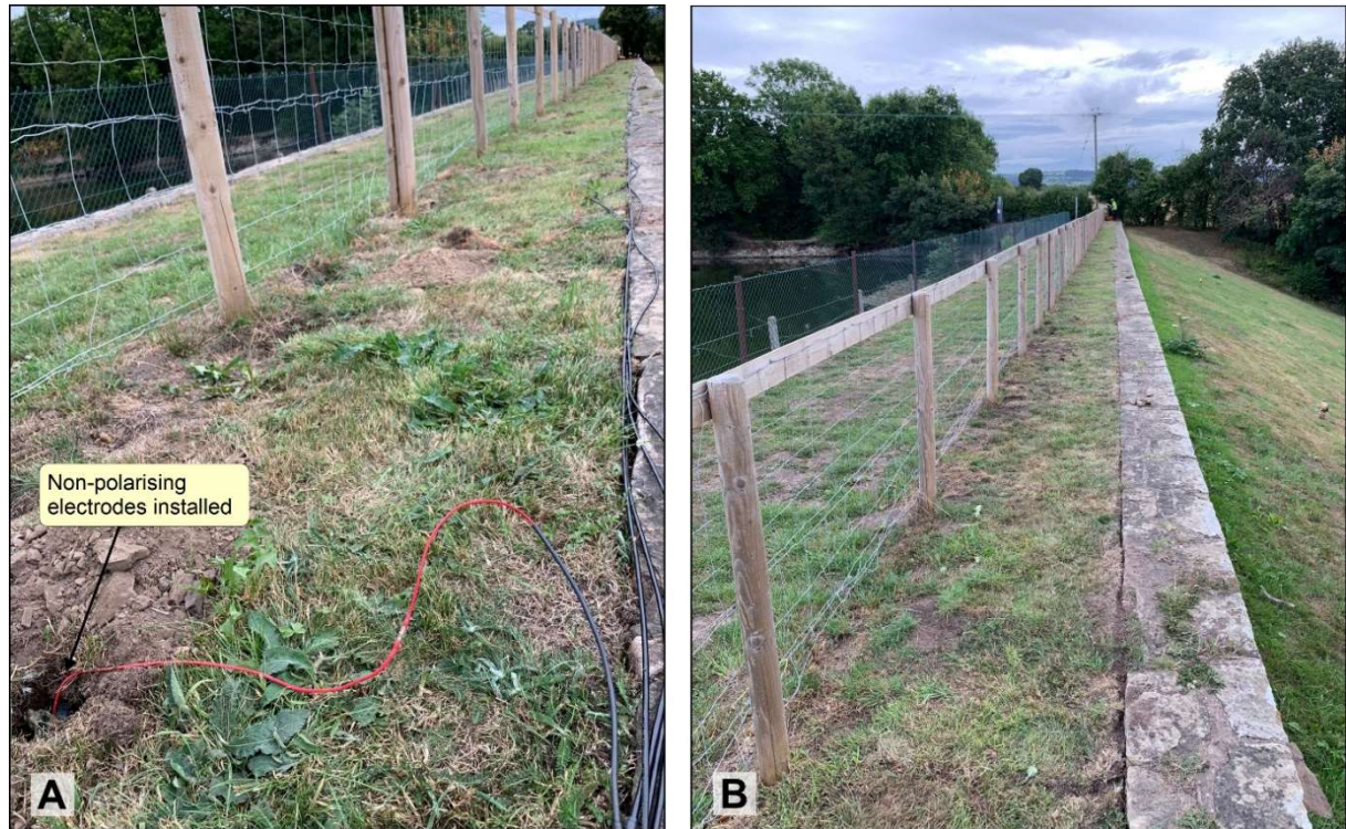
Figure 4. SP monitoring array installation at Oakenholt Reservoir. A) During installation. B) Site conditions following installation.
