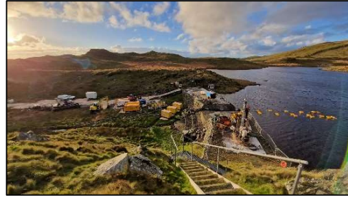
Figure 16. Ground investigation showing access arrangement, ramps, plant and water level management pumping system
