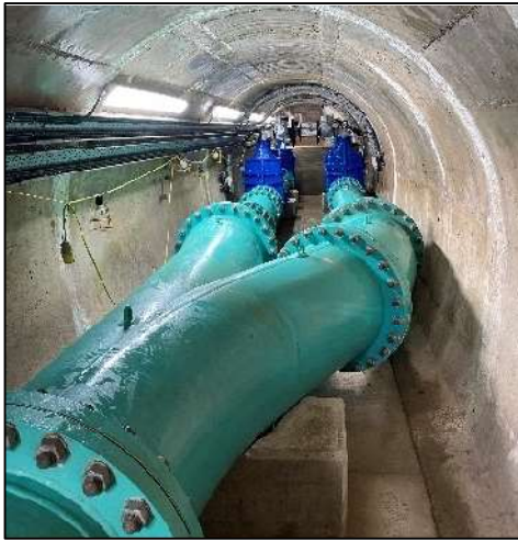
Figure 17. Manifold at bulkhead
