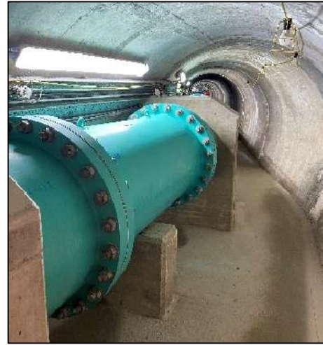
Figure 18. Scour pipework and thrust block
