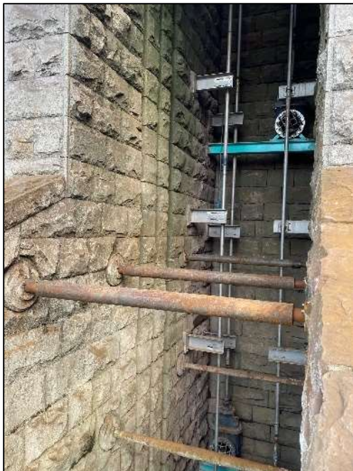
Figure 21. Scour valves and spindles
