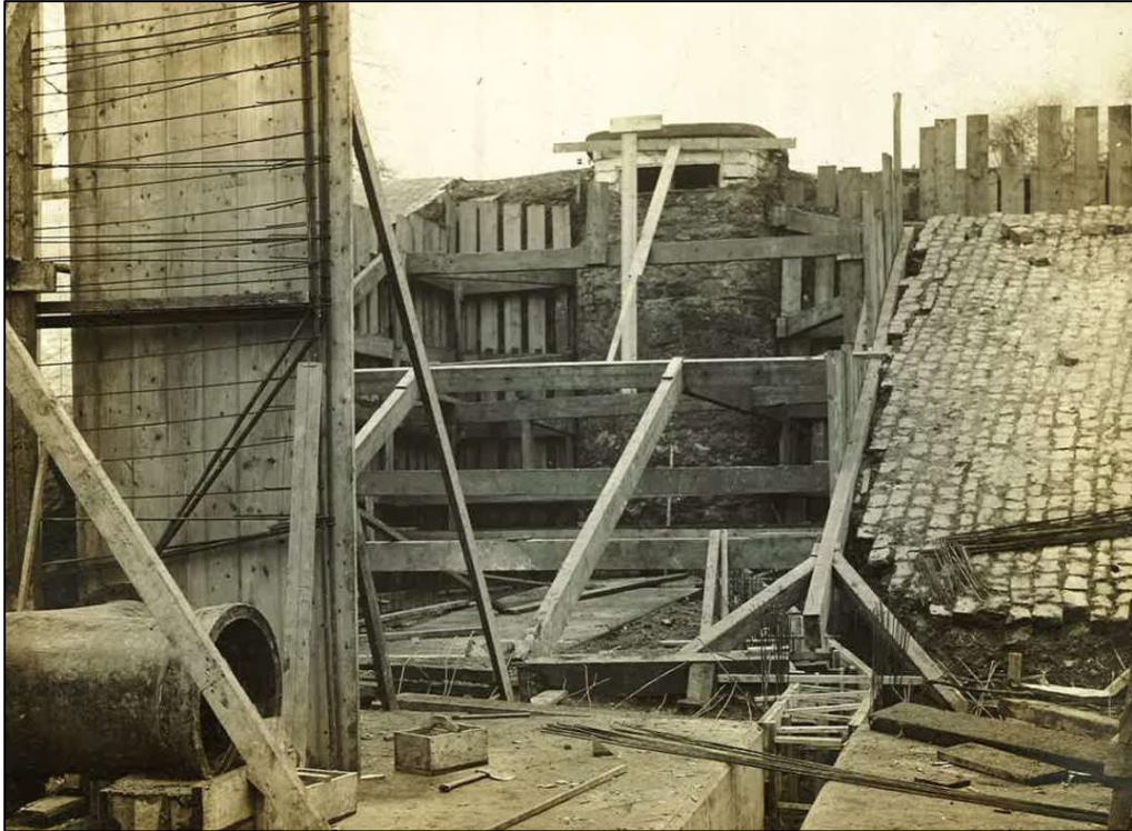
Figure 1. Original open service reservoir with the Engine House and Boiler House in the background.
