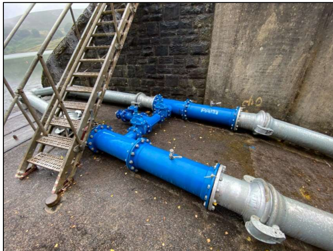
Figure 7. Cwmtillery Reservoir – Siphon priming installation
