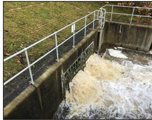
Figure 9. Devil's Bridge Pond – outlet culverts with security screens closed
