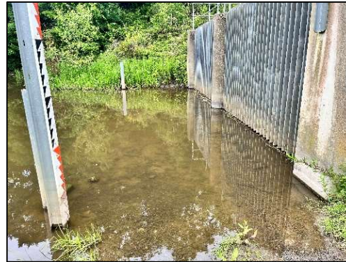
Figure 7. Devil's Bridge Pond – debris screens on inlet of the Hydro-brake™ chamber. Note the concrete invert to aid cleaning of the screen.
