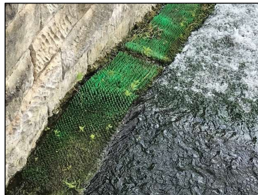
Figure 16. Eel pass installed on a reservoir spillway
