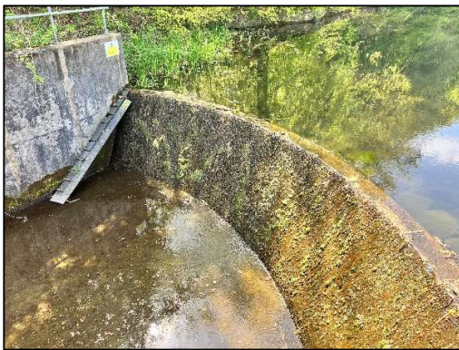
Figure 15. 'Duck' ramp installed on an overflow weir as an alternative to a screen
