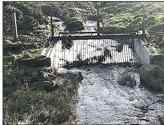
Figure 4. Mammal screen on inlet channel to an amenity lake
