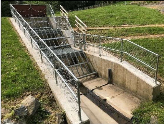
Figure 1. Multi-stage inlet screen to a FSR outlet
