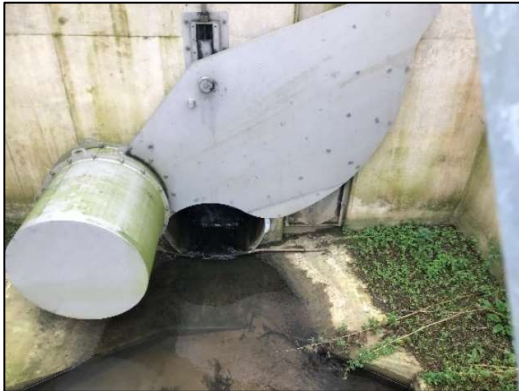
Figure 11. POCFAS – scissor gate at the 1000mm diameter inlet to the FSR control structure (photo taken from inside the debris screen)
