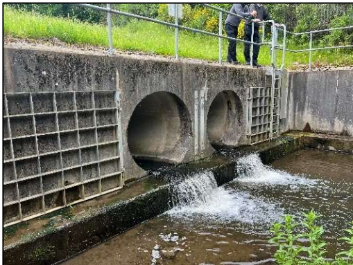
Figure 8. Devil's Bridge Pond – outlet culverts with security screens open
