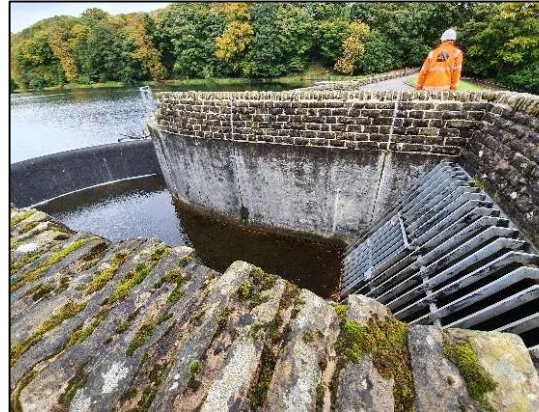
Figure 2. Single stage inlet security screen to a reservoir overflow culvert
