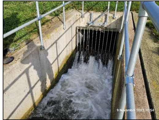
Figure 12. POCFAS – outlet security screen in November 2023
