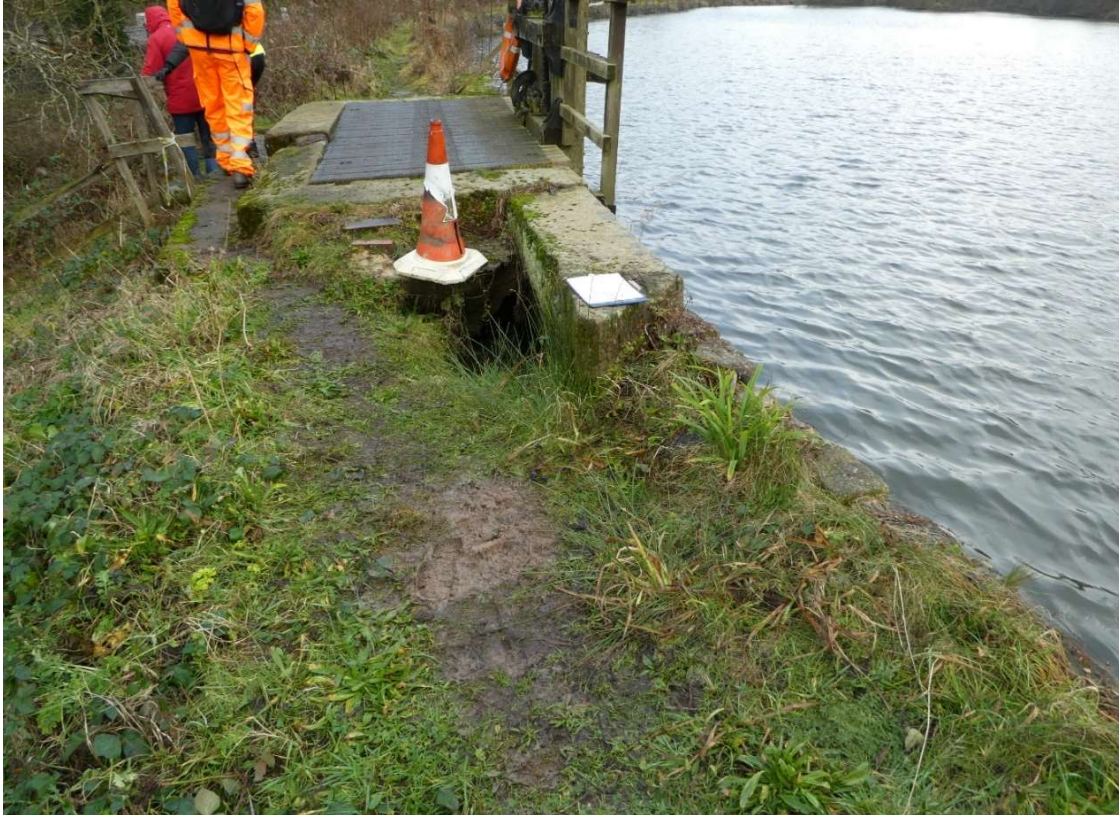
Figure 4. Void within the East Embankment adjacent to the overflow and spillway structure
