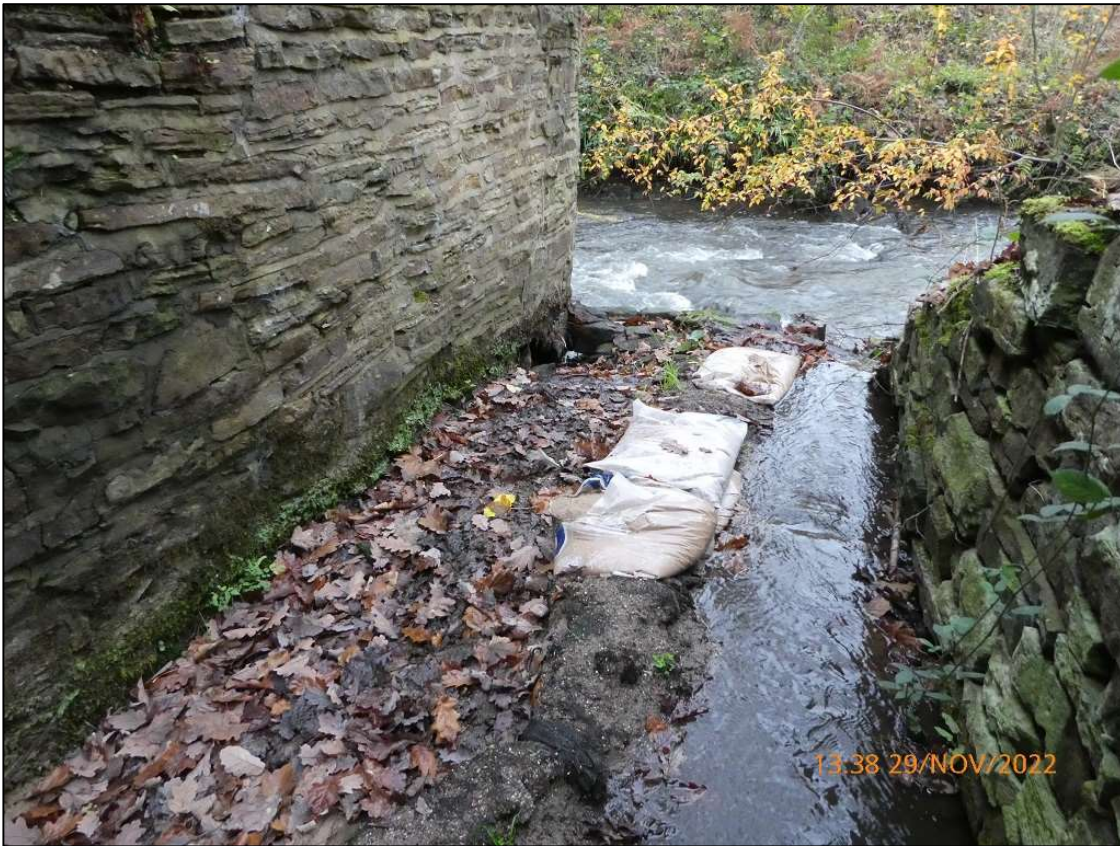
Figure 3. Damage to the downstream end of the spillway channel
