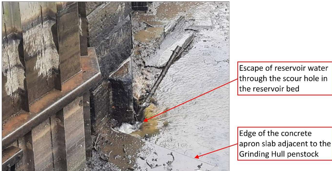
Figure 8. Void in the reservoir basin's puddle clay lining adjacent to the 'Grinding Hull' penstock
