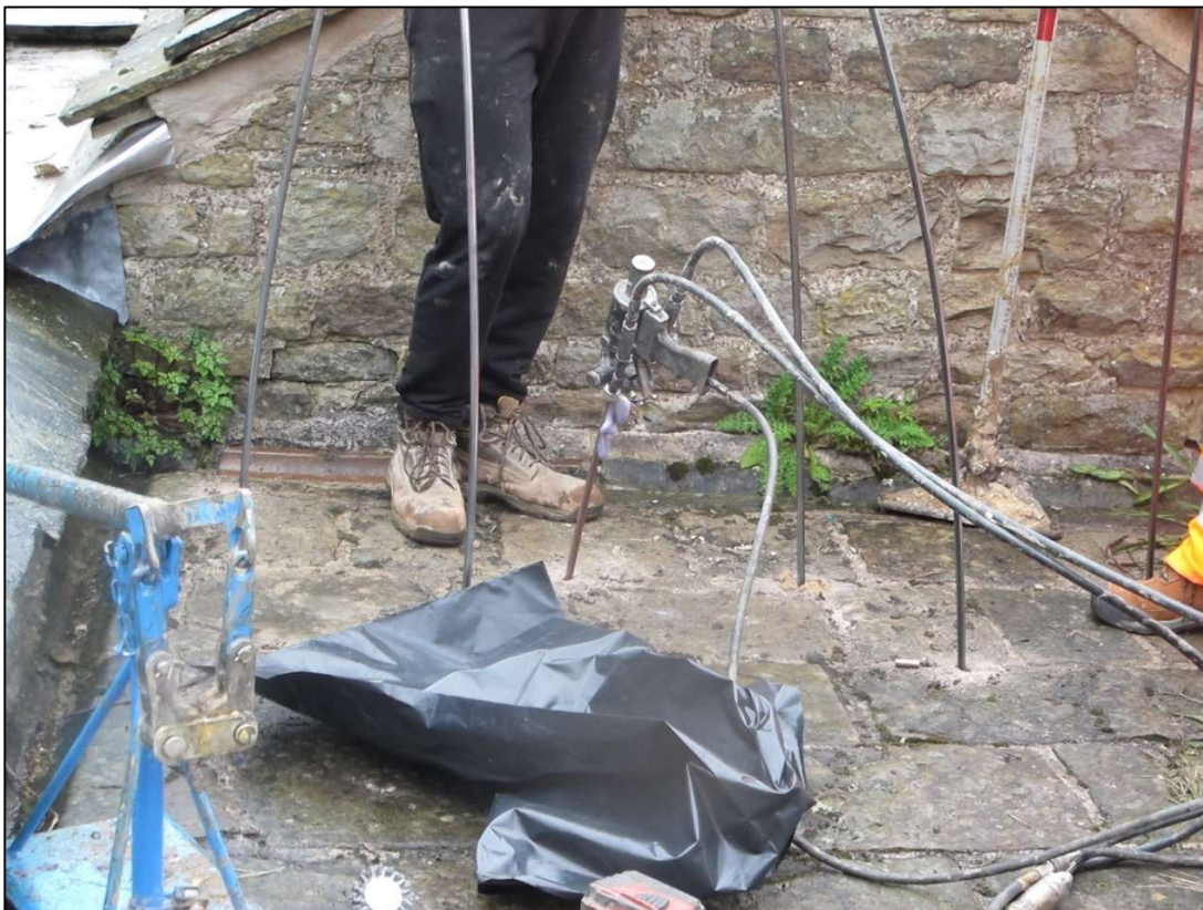
Figure 9. Chemical injection grouting adjacent to the 'Grinding Hull' building (courtesy of Sheffield City Council)
