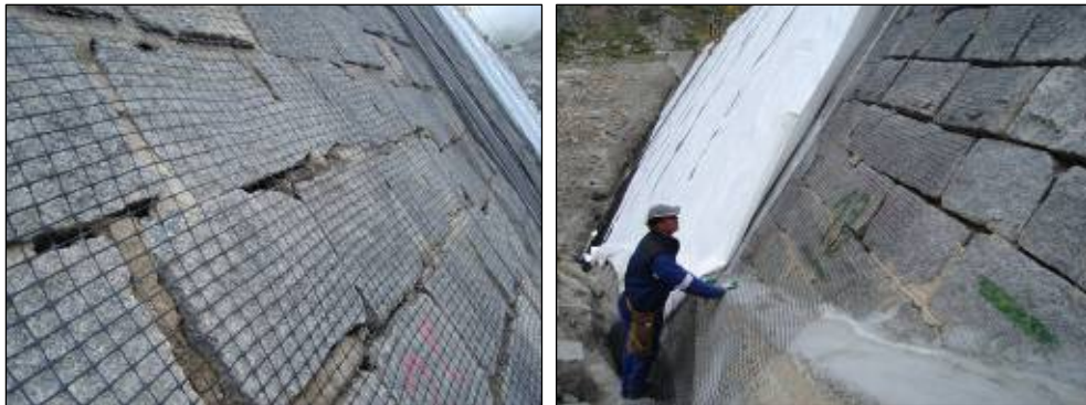
Figures 7 and 8. Support geogrid and anti-puncture geotextile at Karagjol rockfill dam in Bulgaria
