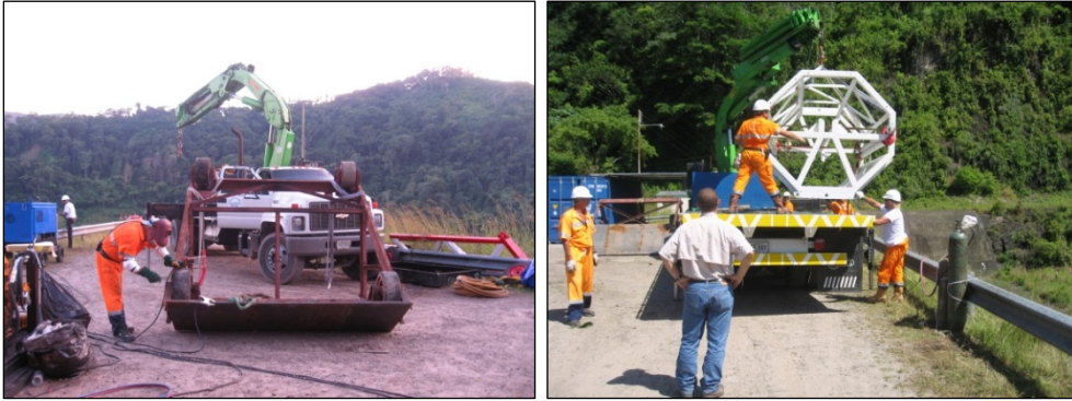
Figures 9 and 10. At left equipment for removal of sediments, at right the structure for placing the waterproofing system, before assembling
