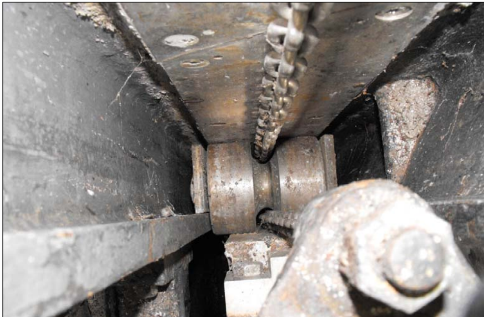
Figure 2. Photograph showing refurbished stainless steel roller train and fixed path.
