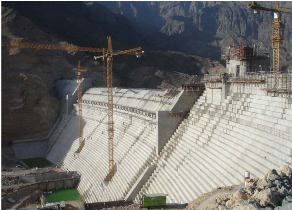
Figure 5: Wadi Dayqah Main RCC Dam downstream face: Last concreting to spillway crest (June 2009)
