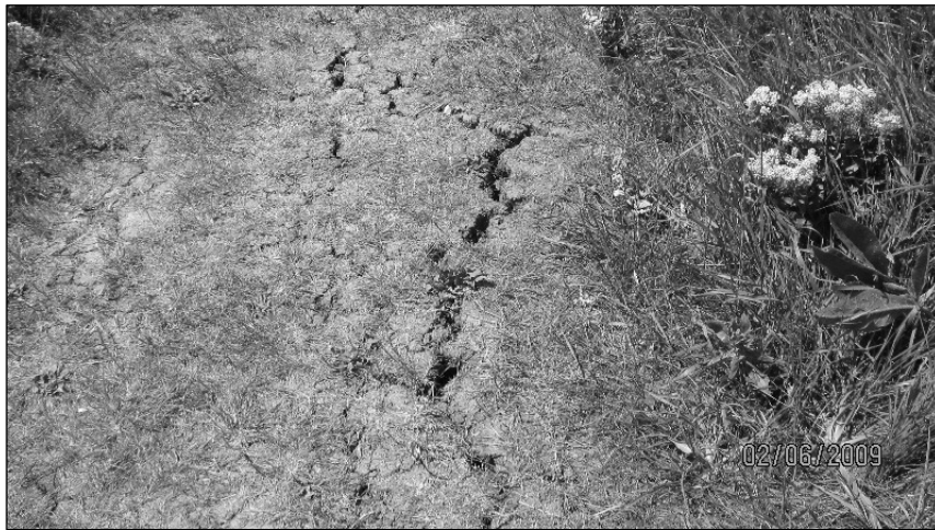
Figure 1. Example of desiccation cracking on flood detention reservoir
