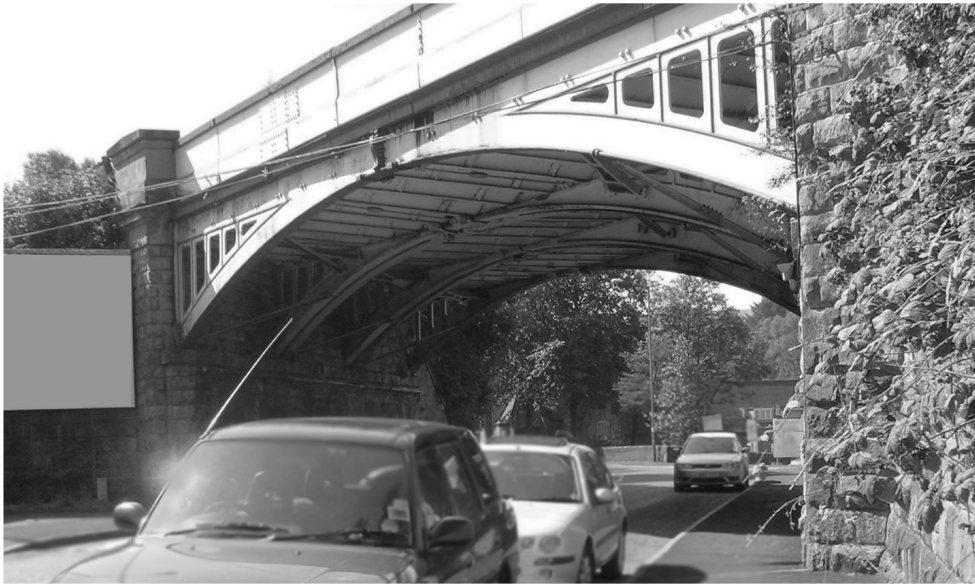
Figure 1: Case History A - Bridge opening through railway embankment
