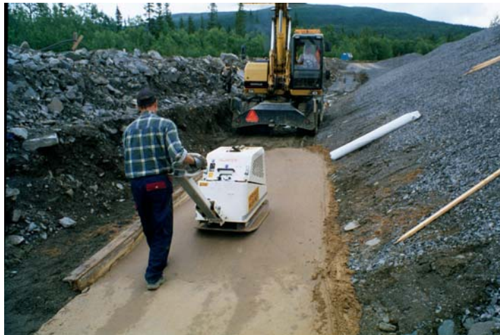
Figure 7. Compaction of the BES bedding layer for the membrane on the existing moraine core. To the right is the compacted coarse filter bedding for the geotextile.
