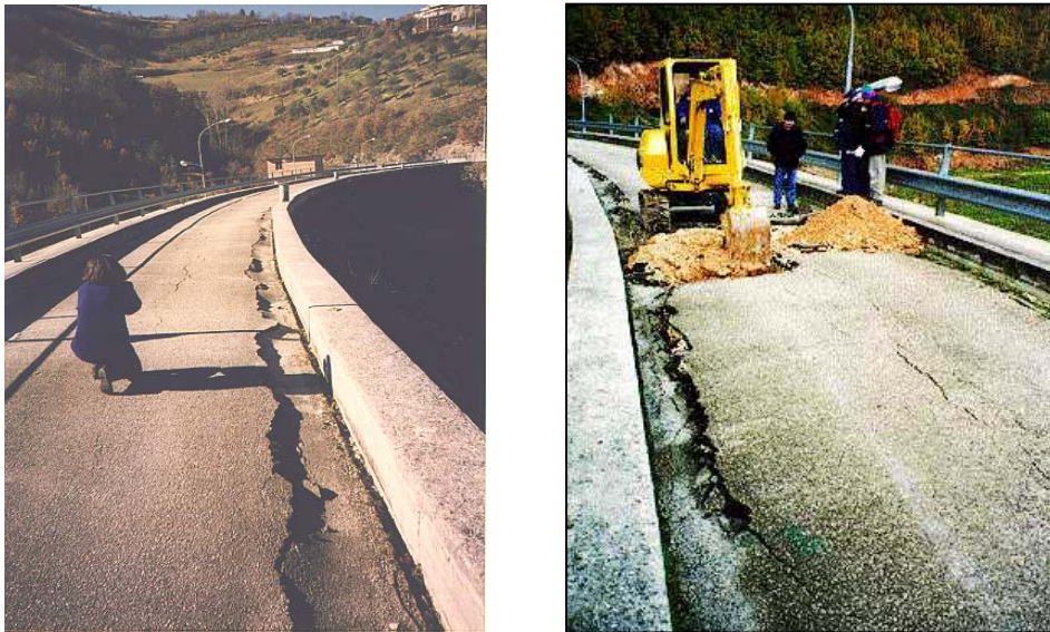
Figure 4. The damage on the crest
