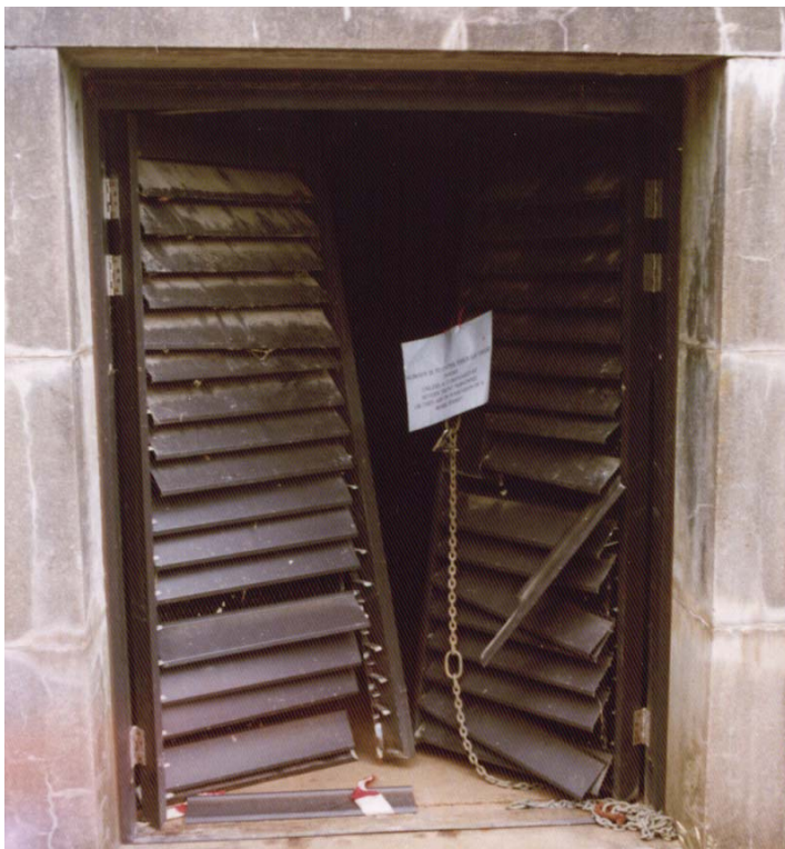
Plate 3: Damaged draw-off tunnel doors
