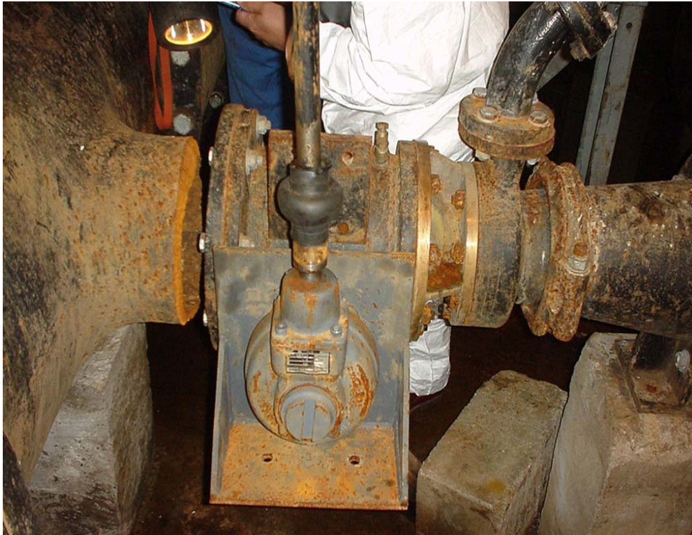
Plate 2: Fractured compensation pipework
