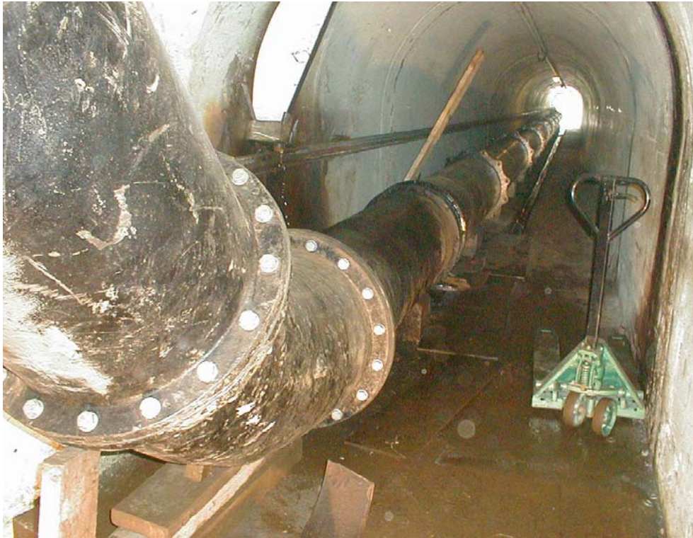
Plate 4: Draw-off main within the draw-off tunnel
