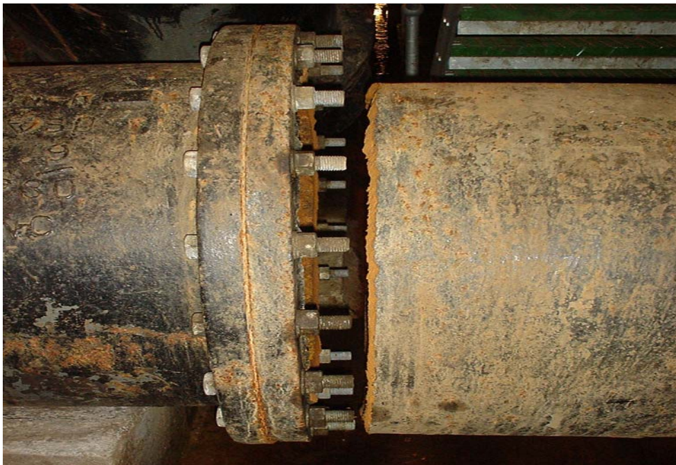
Plate 1: Fractured 30" scour pipe
