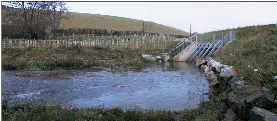
Figure 4: Photograph of inlet arrangement
