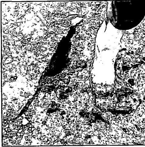
Figure 4 Major defect discovered behind toe beam at chainage 200m
