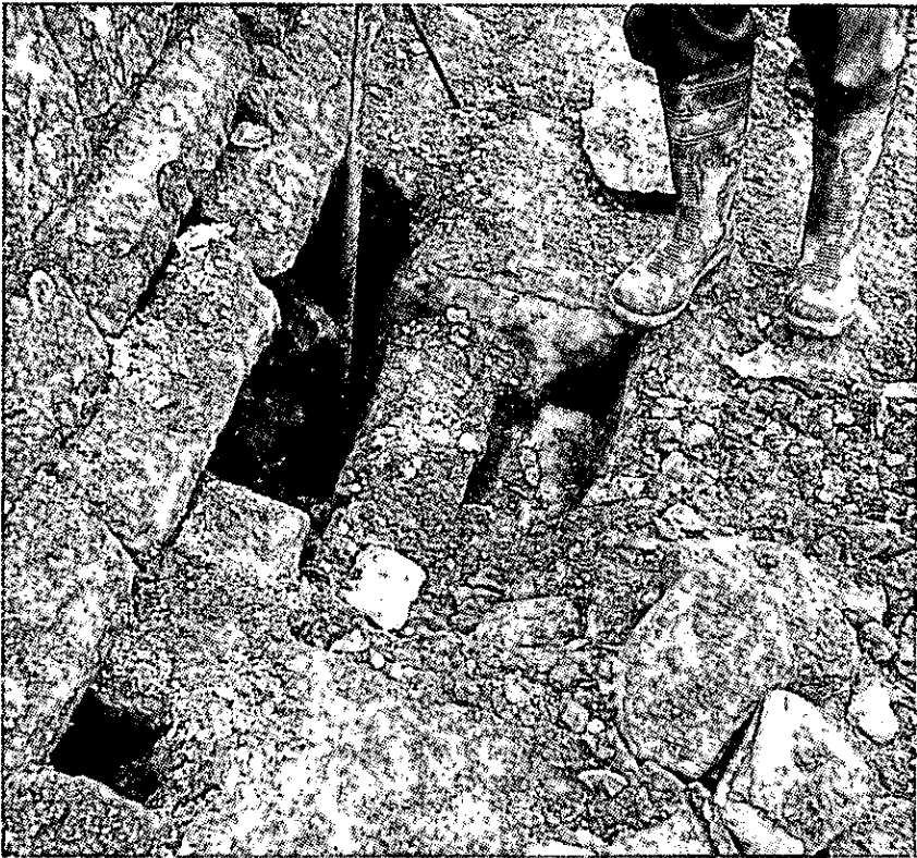
Fig. 3. Hole on the upstream slope of Walshaw Dean Upper dam, 1997
