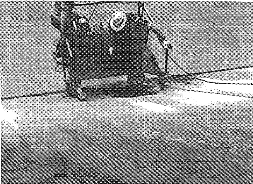
Figure 2 : Repair of a burst blister
