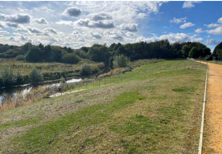
▼ Embankment slope with grass damage
