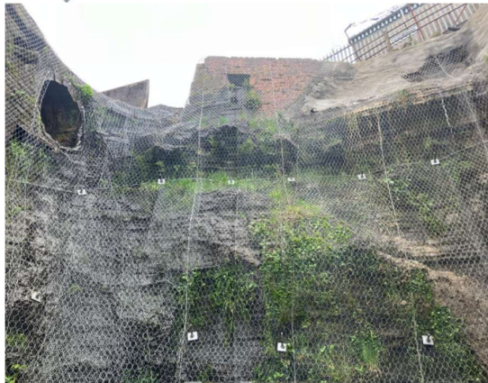
Figure 3 Netting in the Rocky Gorge.
