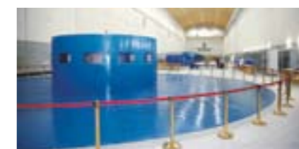
Underground Powerhouse of the 4.8GW Jinping 2 hydropower plant in China.
