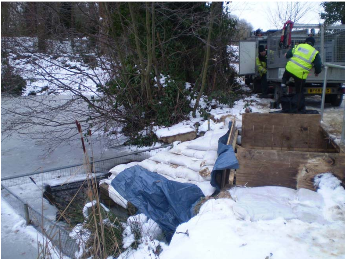
Photo 2: Spillway works at reservoir affected by incident 348
