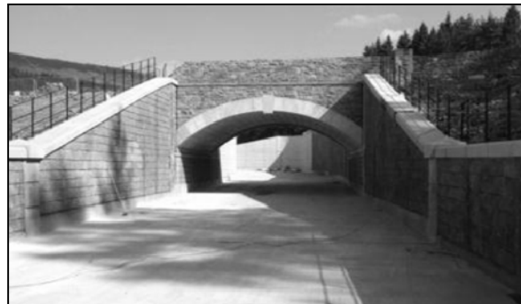
Figure 11. Riding Wood Flexi-arch bridge
