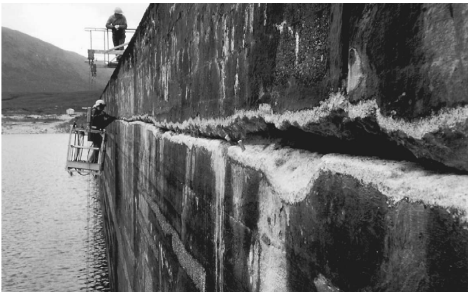
Figure 3 Raked-out joint in upstream face at Blackwater Dam
