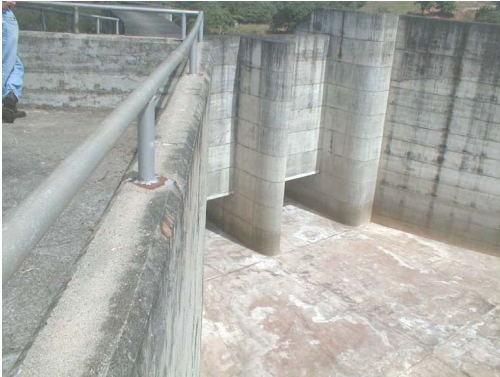
Figure 2. Orifice spillway at 51m high dam. The dam is used partly for flood control
