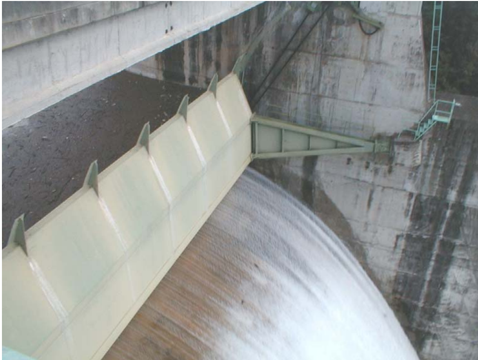
Figure 3. 24 metre long by 5 metre high spillway gate. Synchronization between the two ends is not reliable and the gates are at risk of twisting.
