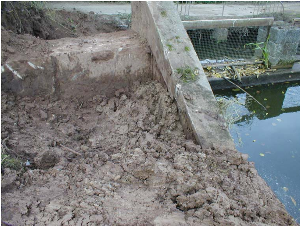
Figure 1. Axial wall on left side of spillway at Upper Hartleton Farm – leakage was taking place beneath the bottom of the wall.
